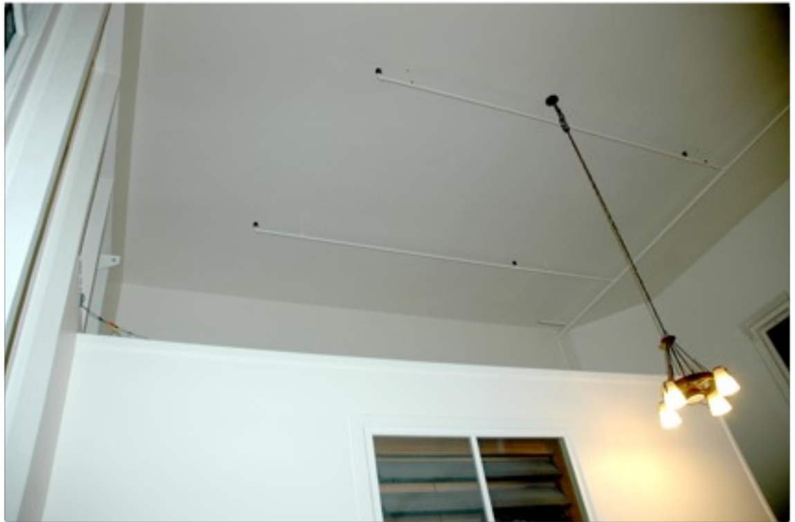
The top of the Pipe room
